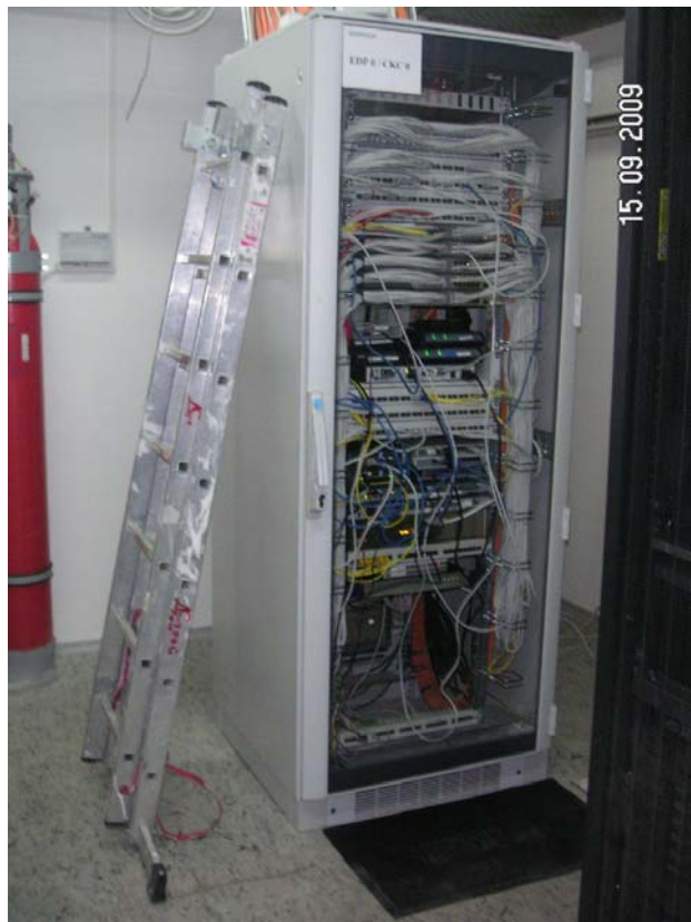
Network Rack at Media-Saturn Stores in Russia
