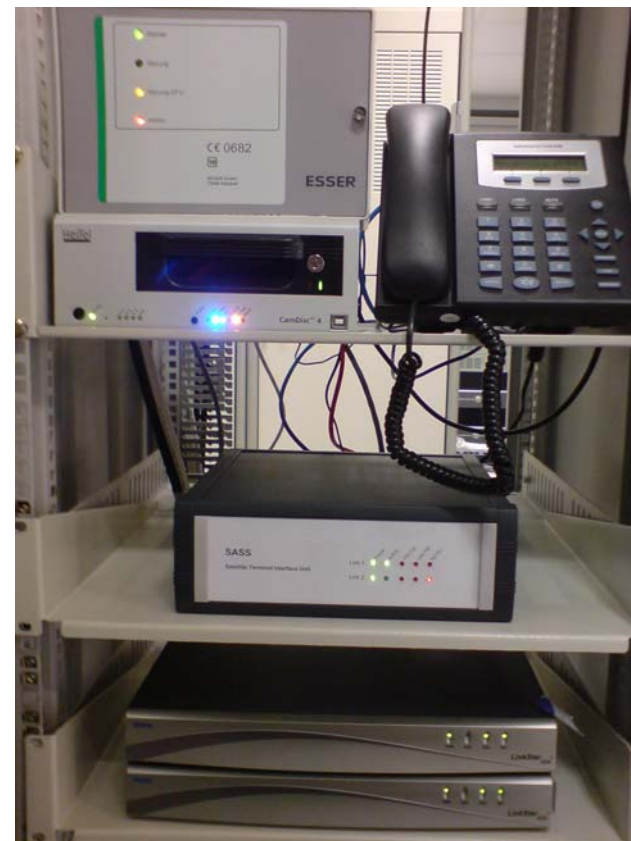
Test Setup at ESRIN Lab in Italy
